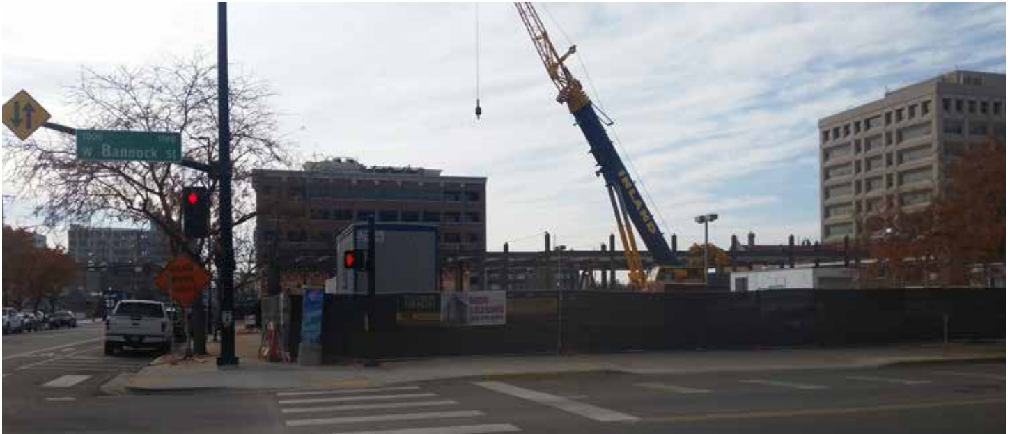
The Westside Park under construction at 11th and Bannock is the type of public space where Current Kinetics could be located, photo courtesy of Arts & History
